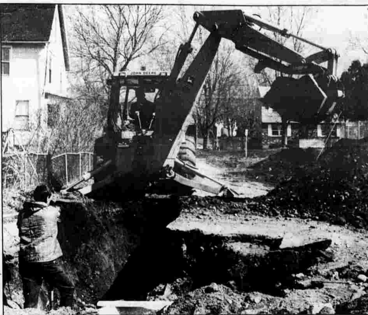
LOWERER SEWER — Town workers Melvin Lobough, operating the backhoe, and Victor Salcius dig a trench in preparation for lowering a sewer line in the driveway to Charter Oak Street from Charter Oak Park. The line must be lowered because part of it will have to go under new culverts.
